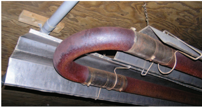
Figure 1.5. Radiant tube heater lacking heat shield. Note close proximity to combustibles (wood ceiling and conduit). (Photo credit: R. Drysdale, Farm Mutual Reinsurance Plan)
