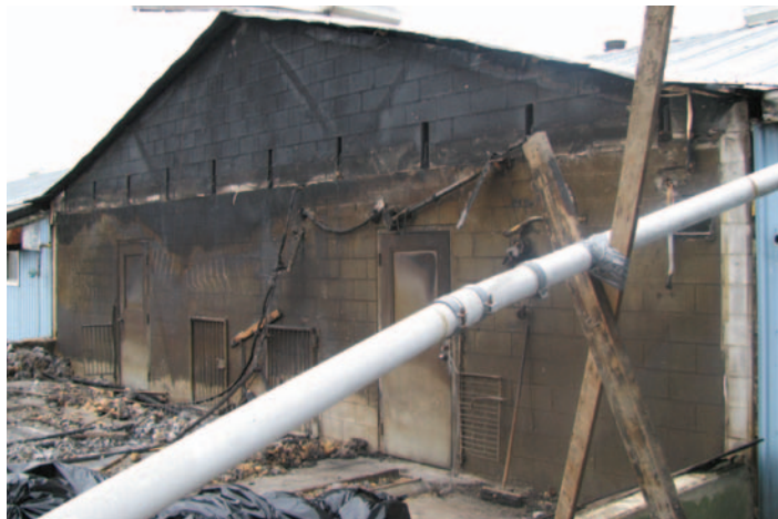
Figure 3.1. Example of a fire separation that served its purpose in a swine complex, preventing the fire from spreading to the rest of the barn.
