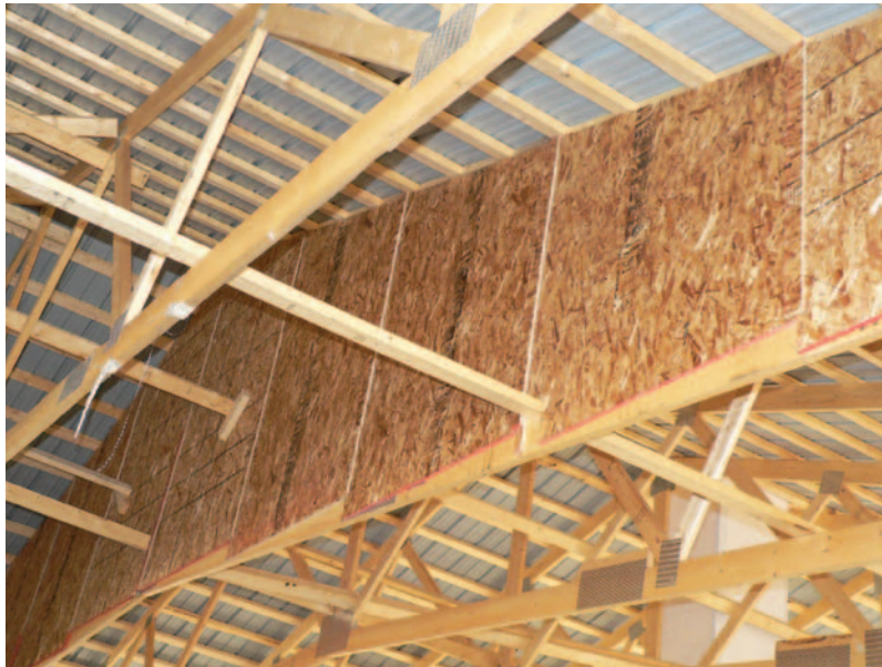
Figure 3.6. Example of an attic fire stop under construction in a new calf barn.
