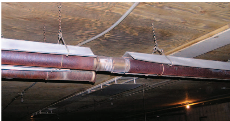
Figure 1.4. Radiant tube heater with heat shield displaced. Note charring on the ceiling.
