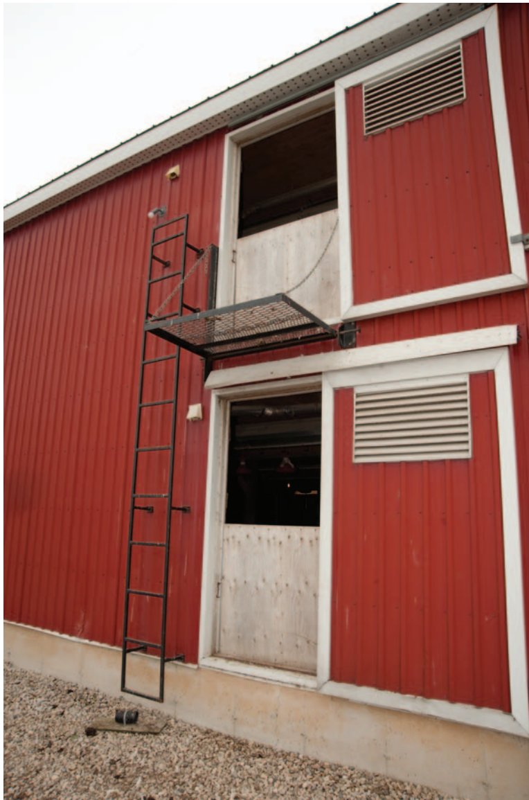
Figure 4.9. An example of a fire exit ladder located beside exit doors on a two storey broiler barn.
