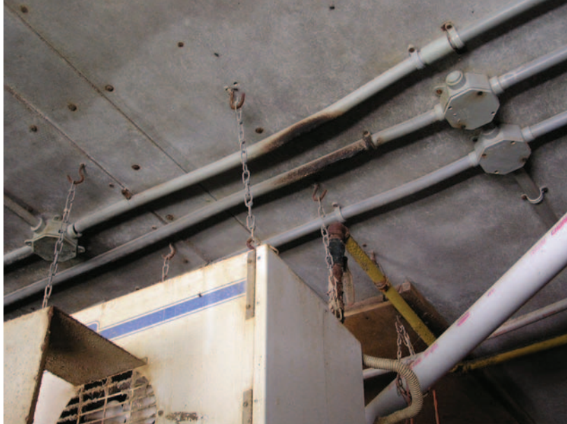
Figure 3.14. A box heater properly suspended on four jack chains. Note that a faulty gas valve resulted in charring of the electrical conduit. (Photo credit: R. Drysdale, Farm Mutual Reinsurance Plan)
