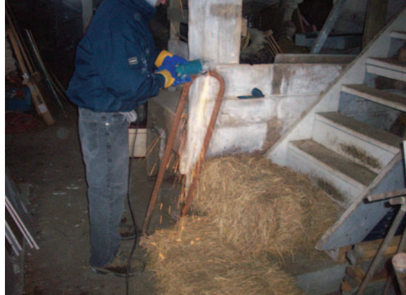
Figure 1.3. Grinding operation taking place in the presence of combustible materials. Use this type of equipment outside the barn and away from combustibles, or put safeguards in place to reduce the risk of accidental ignition.
